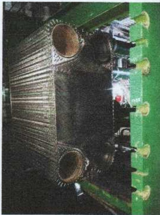
Gambar. Circulating Heat Exchanger
